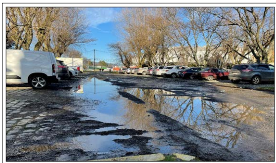
Figure 2: Current Conditions of the Germán Becker Stadium Parking Lot without PICP, City of Temuco, Chile.
