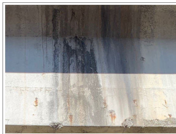
Figure 17: Semi-discovered steel reinforcement as a consequence of the loss of coating, in the structure of the Fig. 11 (photo by the author, taken with a drone).
