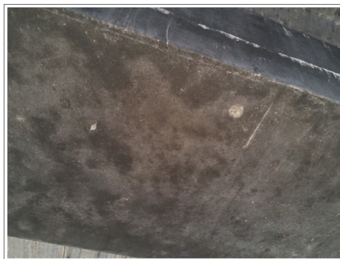
Figure 11: Slight chipping at the bottom flange of a beam, revealing the grey colour concrete (photograph by the author).
