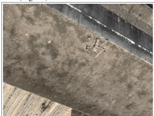
Figure 12: Multi-rotor drone approaching the beams that had suffered a fire, to be able to contemplate what is collected in the Fig. 11 (photograph by the author).
