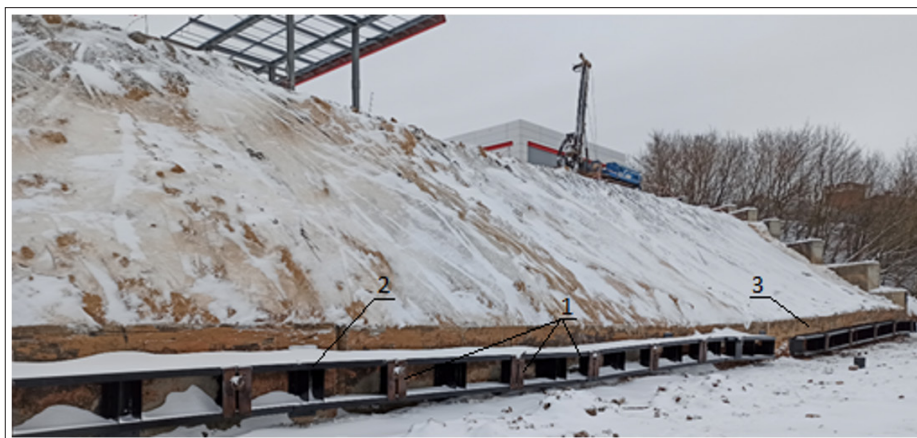
Figure 3: Photograph of the anchoring of the deformed slope on the landslide slope at the absolute elevation. 94.60: 1 - ground anchor; 2 - anchor strapping belt; 3 - corner monolithic reinforced concrete retaining walls.
