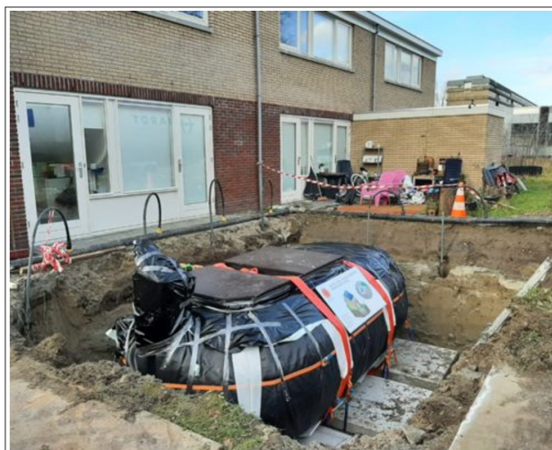
Figure 12: Image of the installation of a Borg-Buffer in a garden at the Green Village
