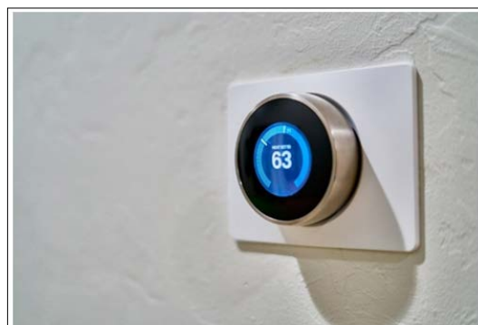
Figure 4: Intelligent Thermostat Installed in a Residential Building US
