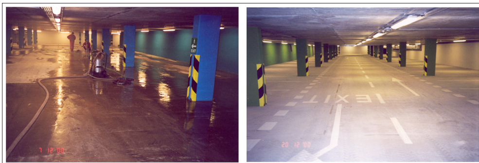
Figure 5: The Lowest Floor of the Underground Garage in Front of the Carlton Hotel After the Water Pumping has been Completed and the Working Joints have been Sealed (Photo by Hulla)
