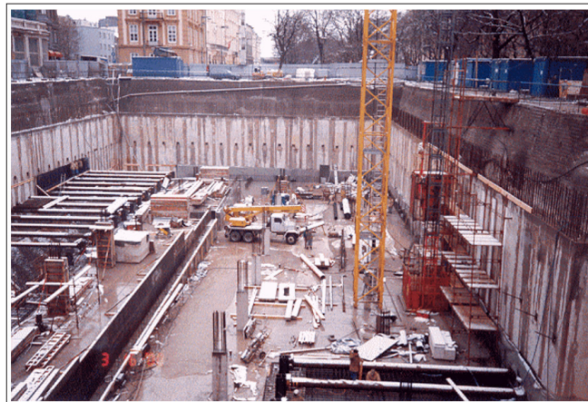
Figure 3: Construction Pit for Underground Garages in Bratislava, in Front of Carlton Hotel (Photo by Hulla)
